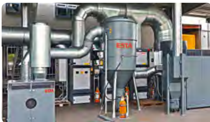
Attachment for welding fume extraction in three production halls at a car manufacturer. Several WELDEX FE cyclone filters, pre-separators and fans
