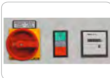
Control panel with operating hour meter
