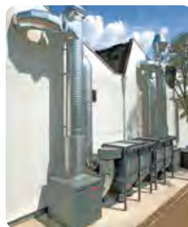
Central extraction systems with two DUSTMAC S filter modules each
